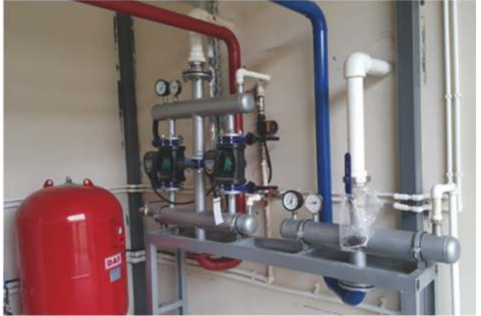
Main Circulation Pumps Collector System
